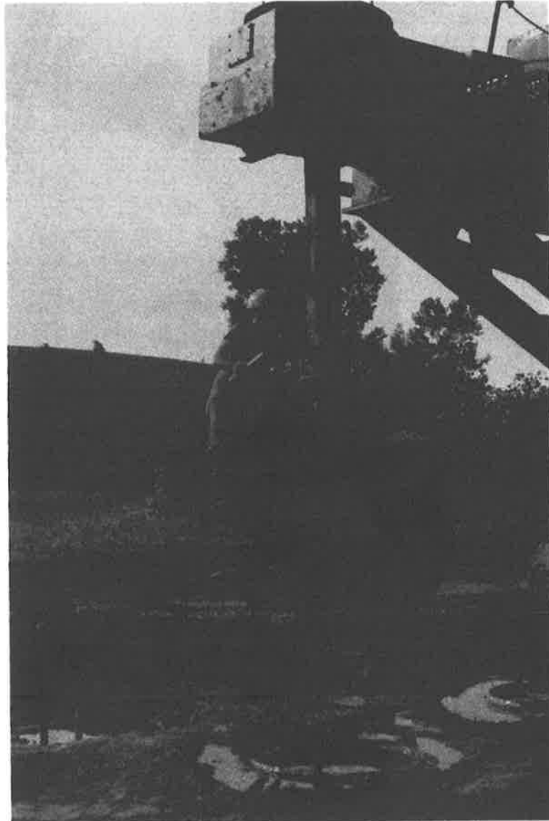
Photo 15 Lining up and leveling of the 5 foot auger to drill the access shaft between the four completed caissons. This view looking south shows the North caisson in the foreground.
