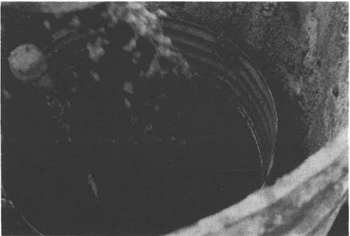
Photo 10 Sloppy-drop free fall of concrete in the East caisson at a depth of 22 to 32 feet using Mix #1 (8.25 inch slump, 1-1/4 inch aggregate and superplasticizer). Note the complete coating of the rebar cage and permanent liner.
