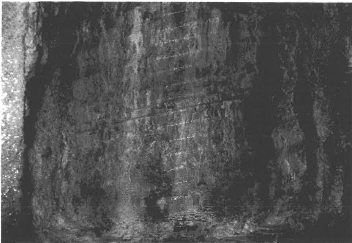
Photo 23 Exposed concrete for the West Caisson as seen through the access shaft Window #3 at a depth of 15 feet below the top of the access casing. Note the wet condition.
