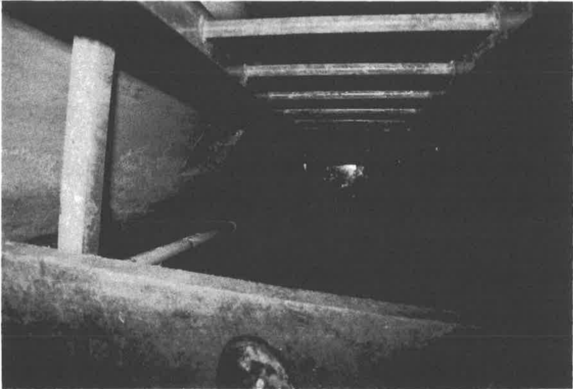
Photo 19 The view inside the access shaft looking down from the platform at window Level 4 at a depth of 30 feet below the surface. after the installation of the ladder, deep well pump, and working platforms. The four windows at Level 5 are visible as is water at the base of the shaft.
