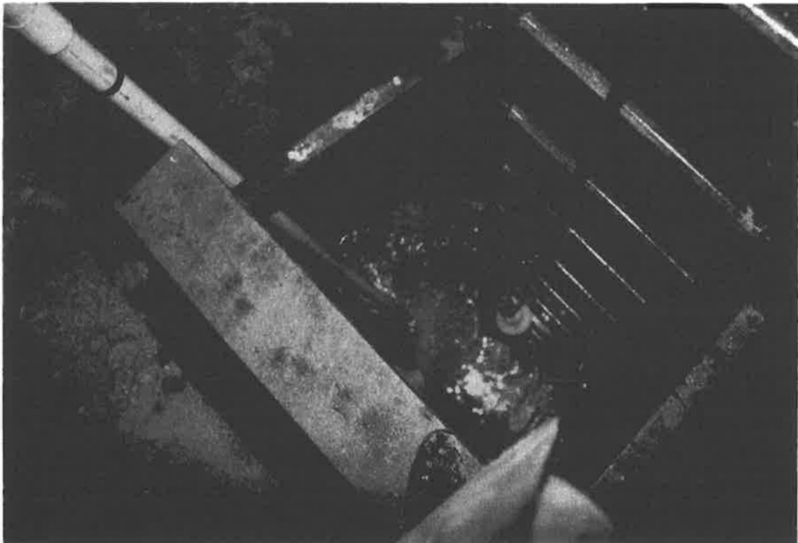
Photo 20 Inside the access shaft at Level 6. Total water infiltration from the upper windows was approximately 1-2 gallons/minute. Here, the water level was pumped down just below the bottom of the Level 7 window. The depth of water was about 6 inches.
