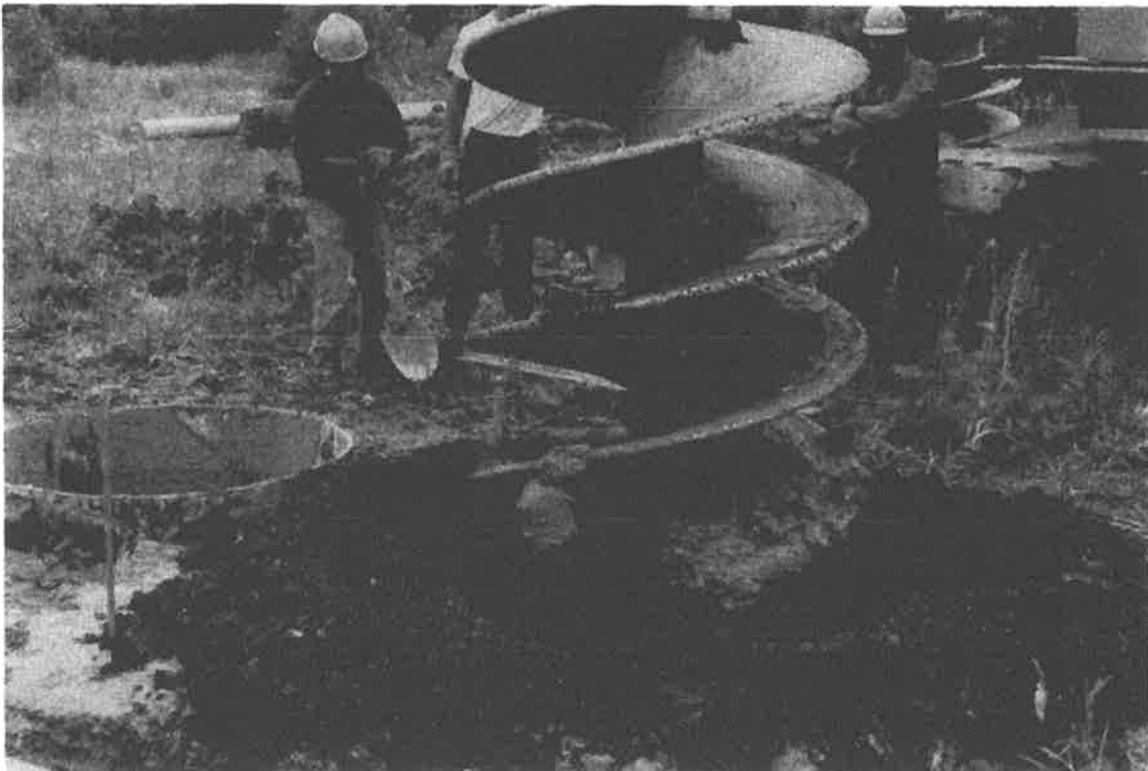
Photo 2 Augering through the rubble fill for the West caisson to set oversize temporary casing.
