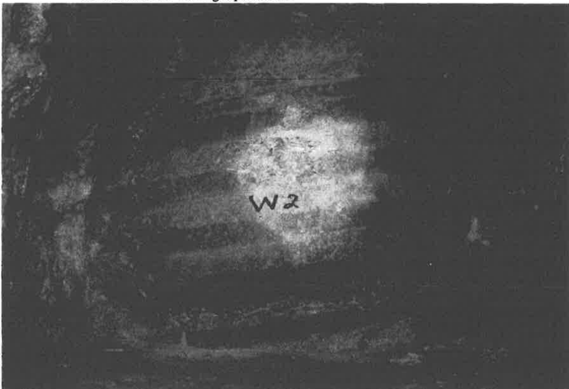
Photo 22 Exposed concrete for the West Caisson at Window Level No. 2, 7 feet below the top of the access casing. Chipping of surface was caused by removal of the corrugated liner.
