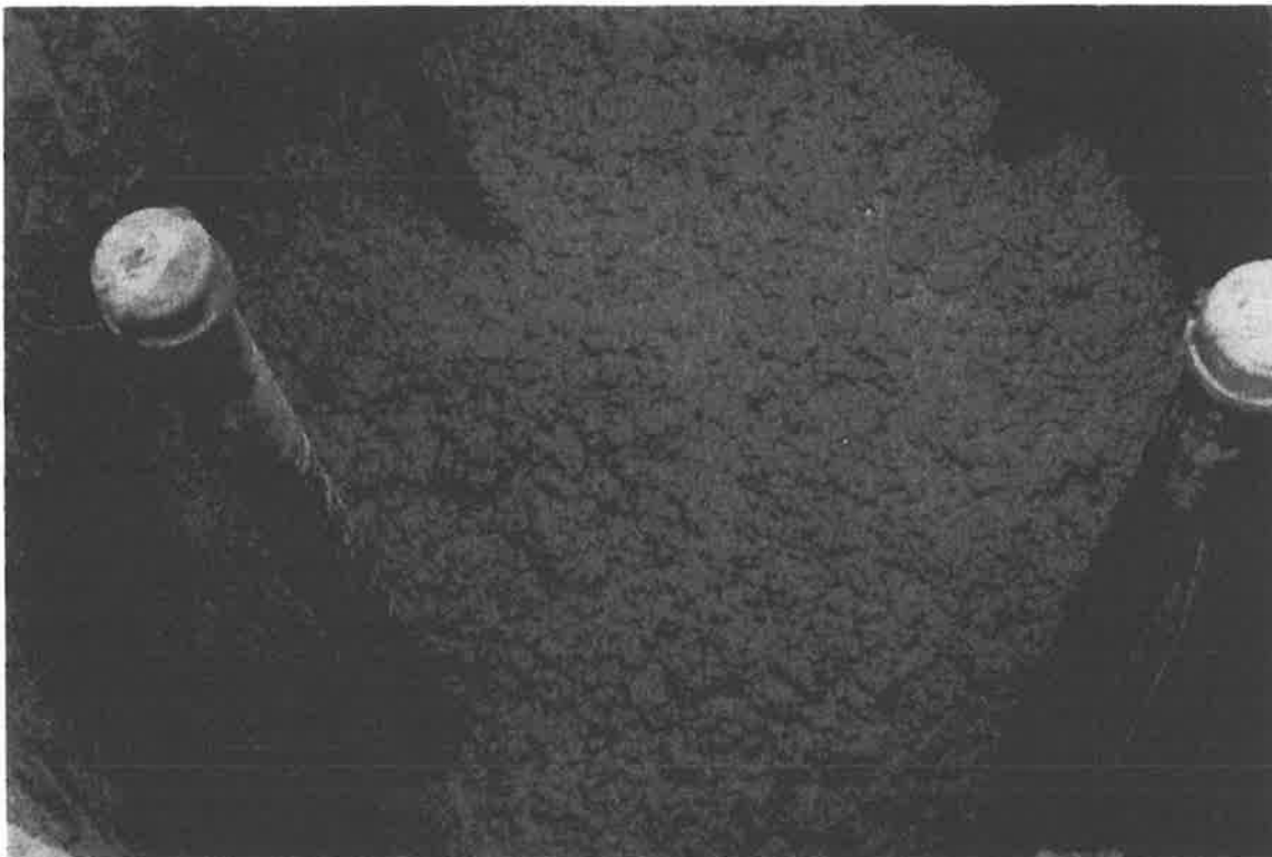
Photo 13 The top of the East caisson just prior to the start of vibrating to a depth of about 2.5 to 3 feet. The top lift was Mix #4 with a 7 inch slump and 5/8 inch aggregate.
