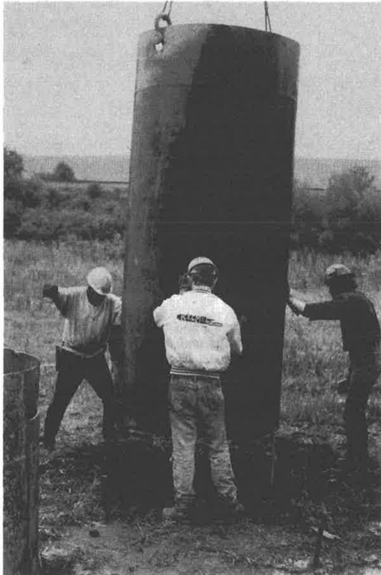
Photo 3 Placement of a 48 inch diameter temporary oversize casing through fill soils for the South caisson.
