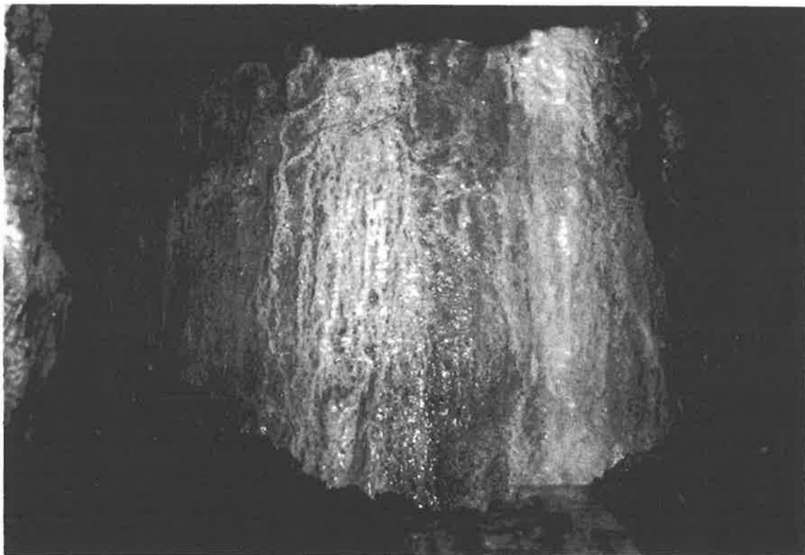
Photo 24 Exposed concrete for the West Caisson at Window level #4 at a depth of 25 feet below the top of the access casing. The concrete is fully formed while somewhat rough. No segregation, voids or honeycombing is evident.
