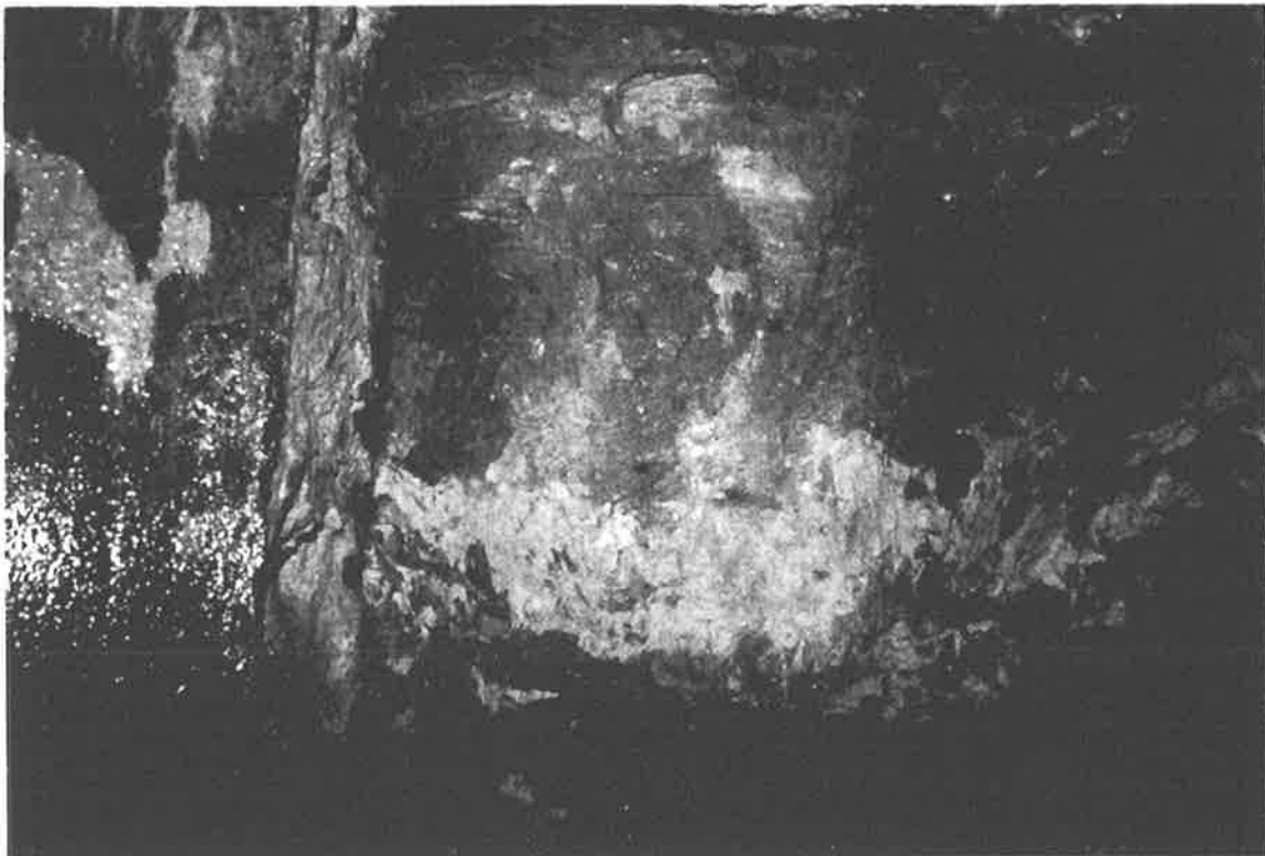
Photo 26 Exposed concrete for the West Caisson at Window Level #6 at a depth of 45 feet below the top of the access casing. The white muck on the surface are concrete cuttings from the coring operation at the surface. The concrete is rough and was chipped during removal of the soil, however, no voids or honeycombing are evident.
