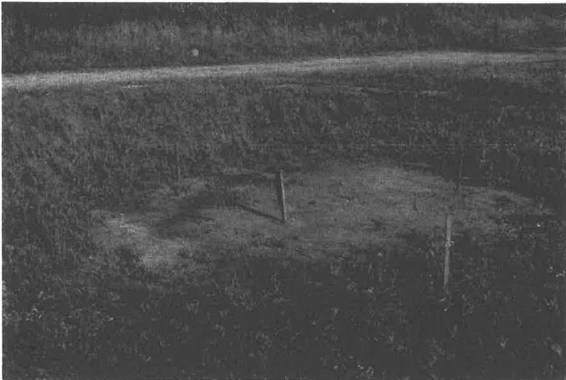
Photo 1 Layout of the four caissons and center access shaft at the project site. The 3 foot diameter shafts and 5 foot diameter access shaft were placed to maintain an approximate 1 foot edge-to-edge clearance.
